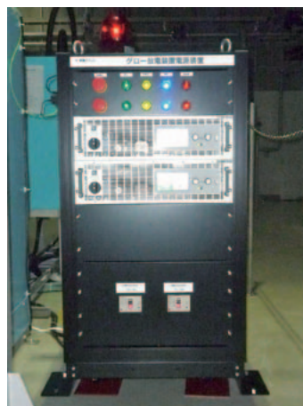
Fig. 4 New power supply for glow discharge cleaning system in LHD
