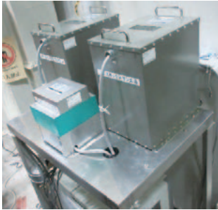
Fig. 1 Two noise cut transformers for Thomson scattering system
