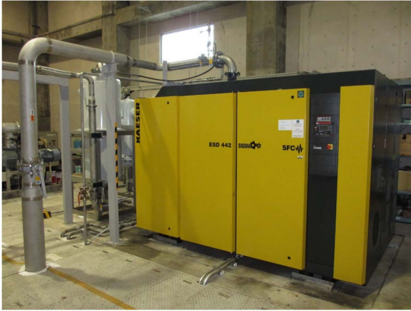
Fig. 1. Photograph of the new main compressor. The oil removal system is installed beyond the compressor.
