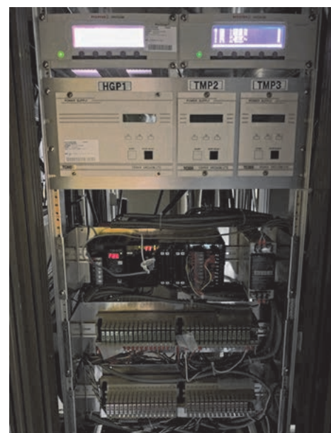
Fig. 20 PLC and controllers of the TESPEL#4.
