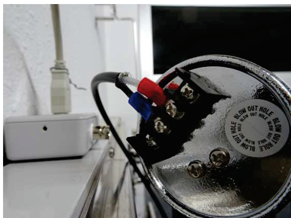
Fig.5: Connection with a pressure gauge
